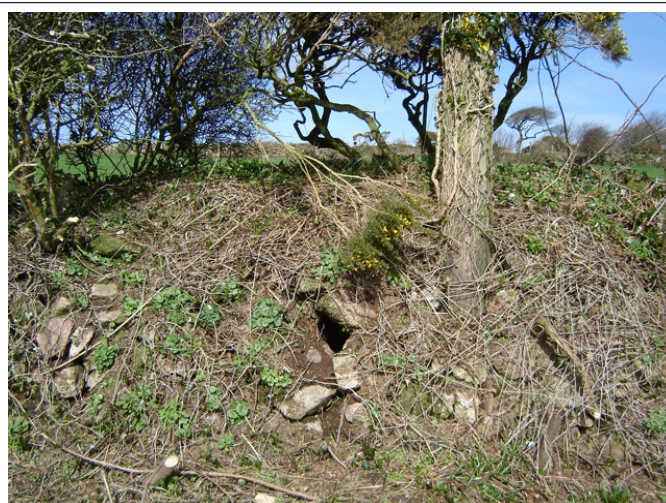
A rabbit-hole like this in the side of a Cornish hedge is easily blocked with a stone to discourage entry. Repeated blocking causes rabbits to move out.
